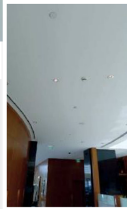
The core of the system was changed, but the speaker circuits remained the same
