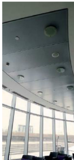
The PA/VA retrofit in the office tower
